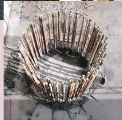
已完成高壓水力清洗的樁頭部份 Pile head after completion of Hydro-demolition
