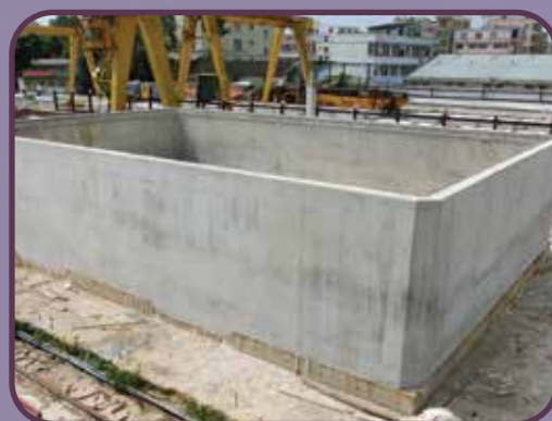
已完成的樁帽殼準備由預製件廠房 運往香港地盤進行安裝 The completed pile-cap shell will be delivered from off-site yard to Hong Kong for installation
