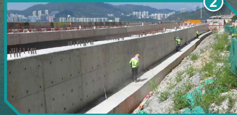
興建地面路段的底層結構 Construction of substructural works at at-grade road section
