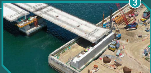
安裝預製箱形橋樑在D9路橋台上 Installation of precast box girder on the abutment at Road D9
