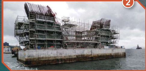
於將軍澳灣現場建造V型橋墩 Cast-in-situ V-pier at Junk Bay
